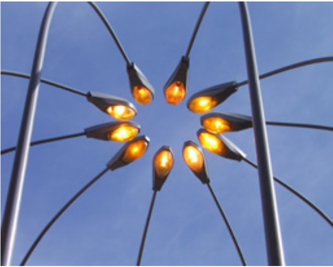
Street lighting as an example of field application to optimise parameters of external lighting
